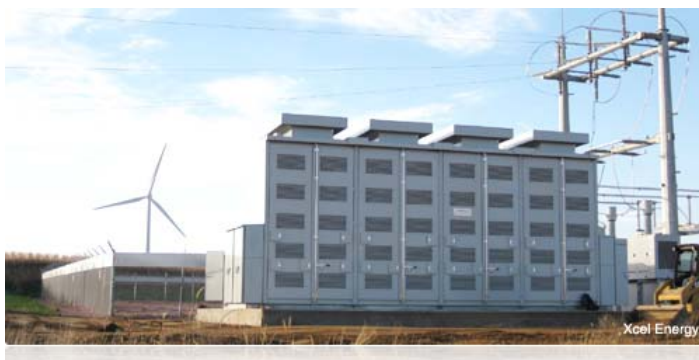
Figure K-3 Sodium-Sulfur Batteries
